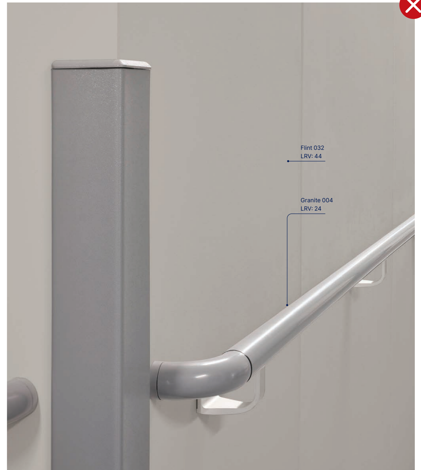
Image shows less than 30 LRV points difference between the handrail and wall
